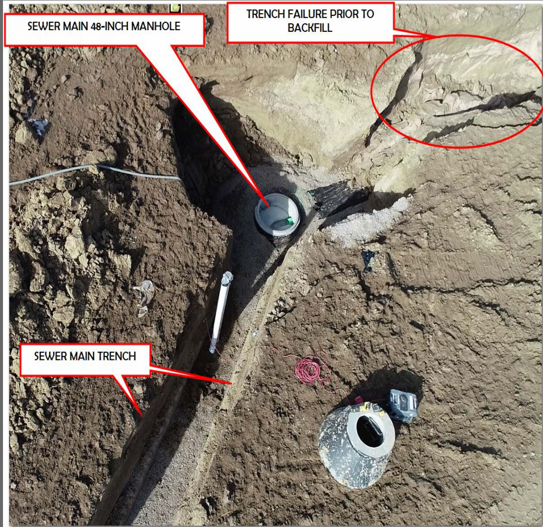
Millstone @ Columbine – Trench Failure Will require manholes be lined
