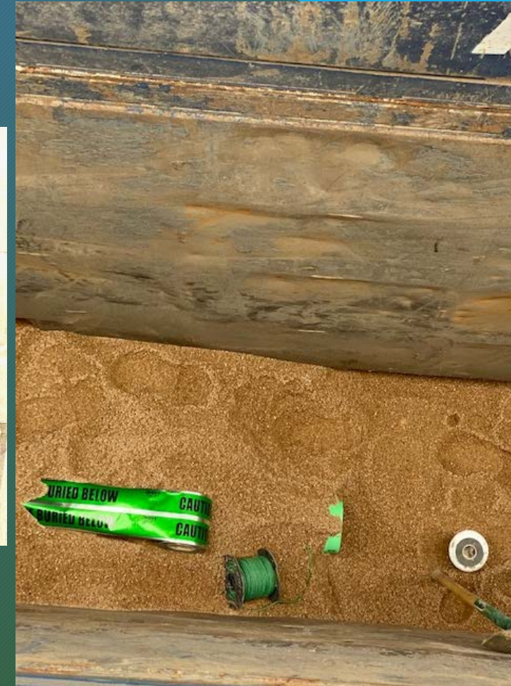
Trace Wire on Sewer Service
