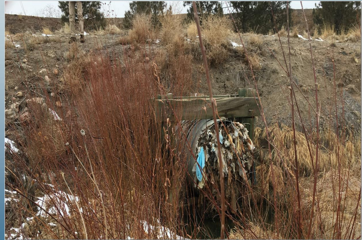
Clogged Storm Drain Downstream of Landfill
