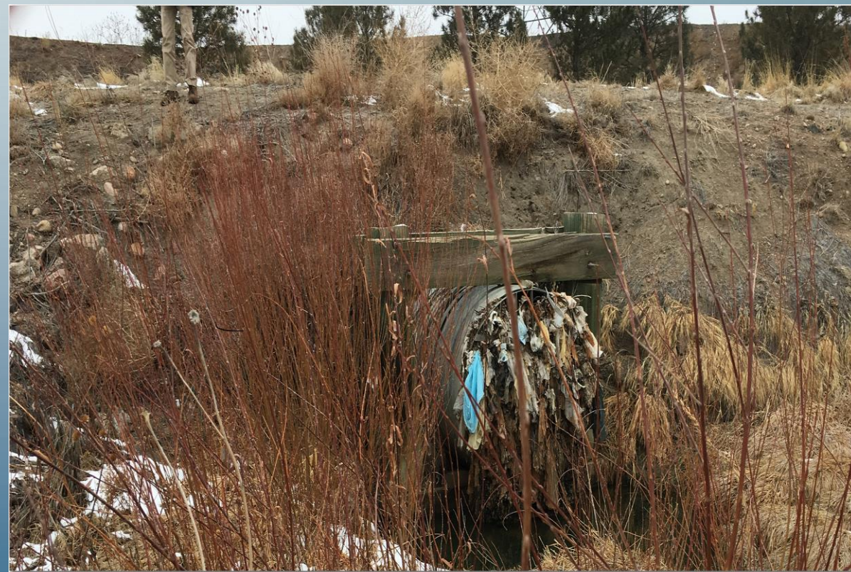
Clogged Storm Drain Downstream of Landfill
