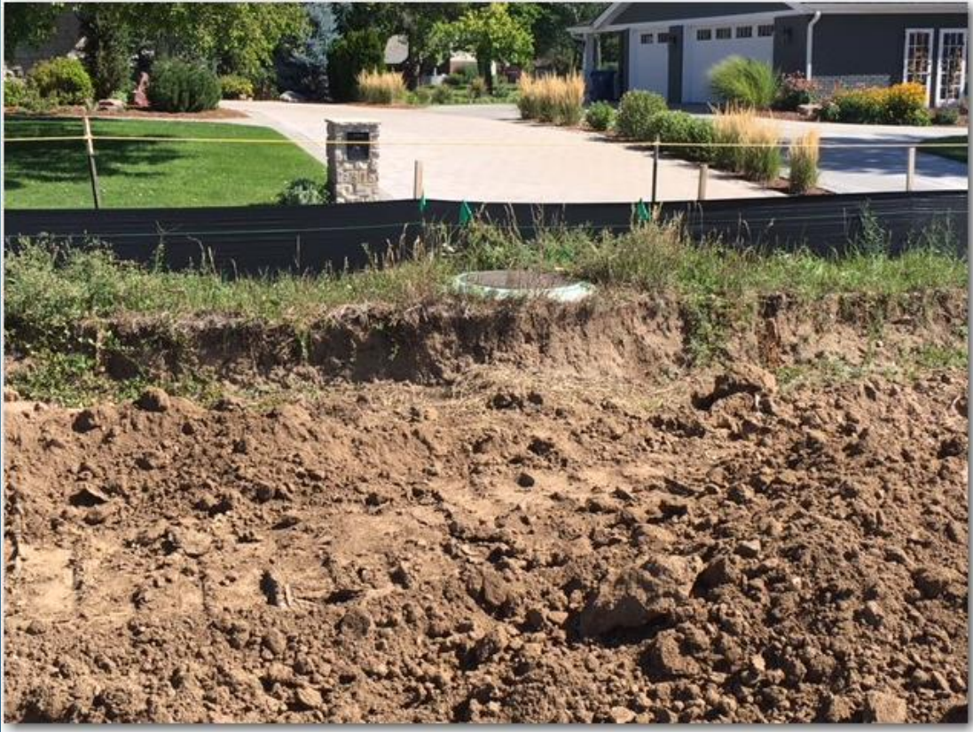
Existing B-Line Manhole 18" Above Grade – Design in Progress
